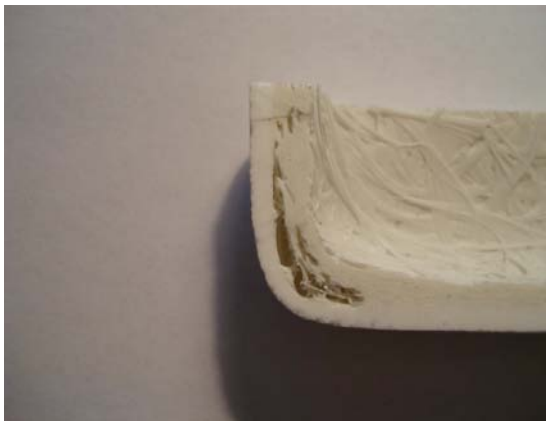
Fig. 1. The sample of the defect in corner
